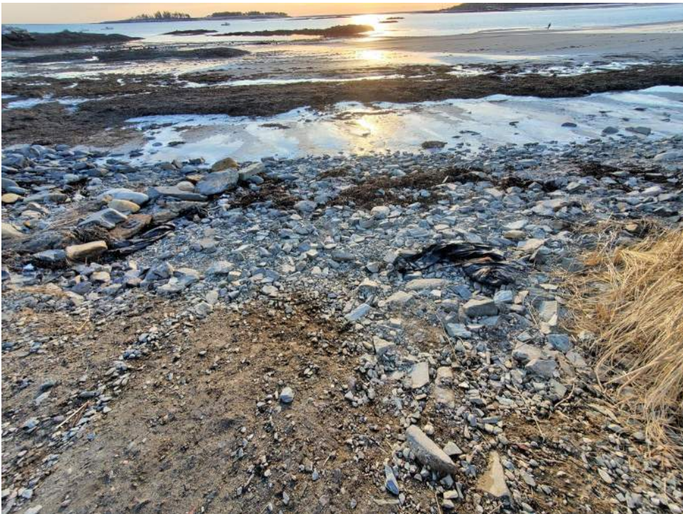
Photo 4 (01/09/2020): Toe of existing watercraft launch area and displacement of gravel and riprap are shown in this image.
