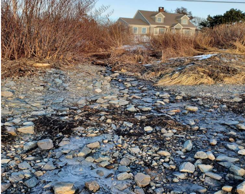
Photo 5 (01/09/2020): Manmade drainage swale (RP-2 Wetland A) located between existing and proposed watercraft launch areas.
